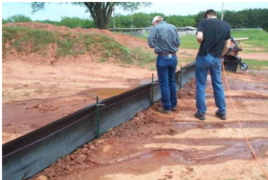
Figure 11 No undercutting of toe of fence – water did pass through fence
