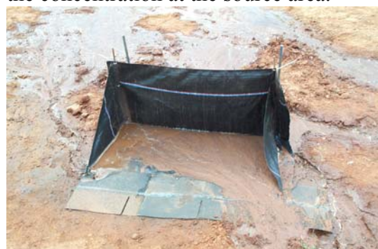
Figure 3 Sediment accumulation between flow barriers
