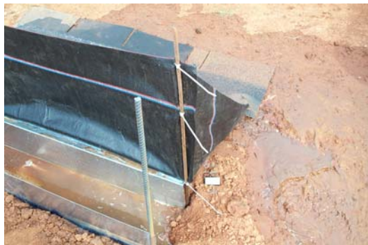
Figure 2 Water flowing through fence and down the side of the trough is relatively
