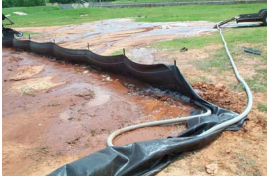
Figure 10 Running water along toe of fence
