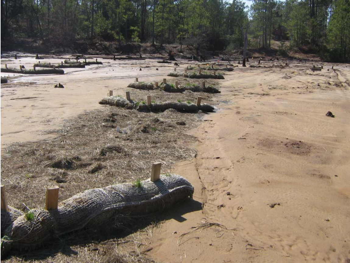
Figure2. Fiber rolls installed and partially planted on an historic brine scar in south Arkansas.
