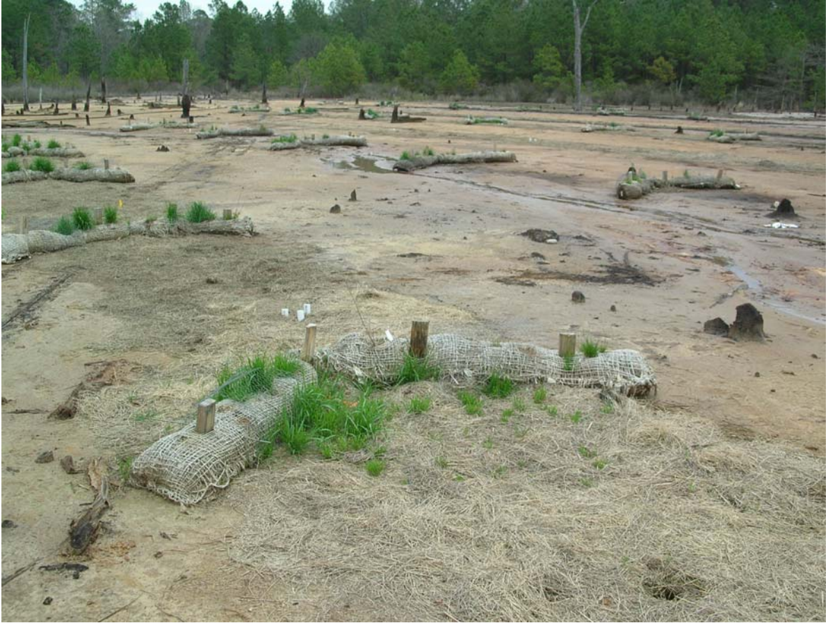
Figure 1. Fiber rolls ca. 20 weeks after planting. Rolls are located in an historic brine scar in south Arkansas.
