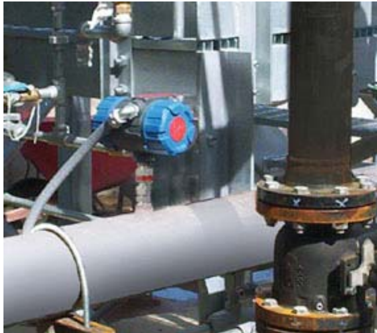
Figure 4 Non-incendive installation of TA2 Thermal mass flow meter for natural gas
