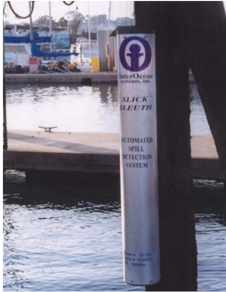
Figure 3. Prototype spill sensor. Installed near fuel pier (background).
