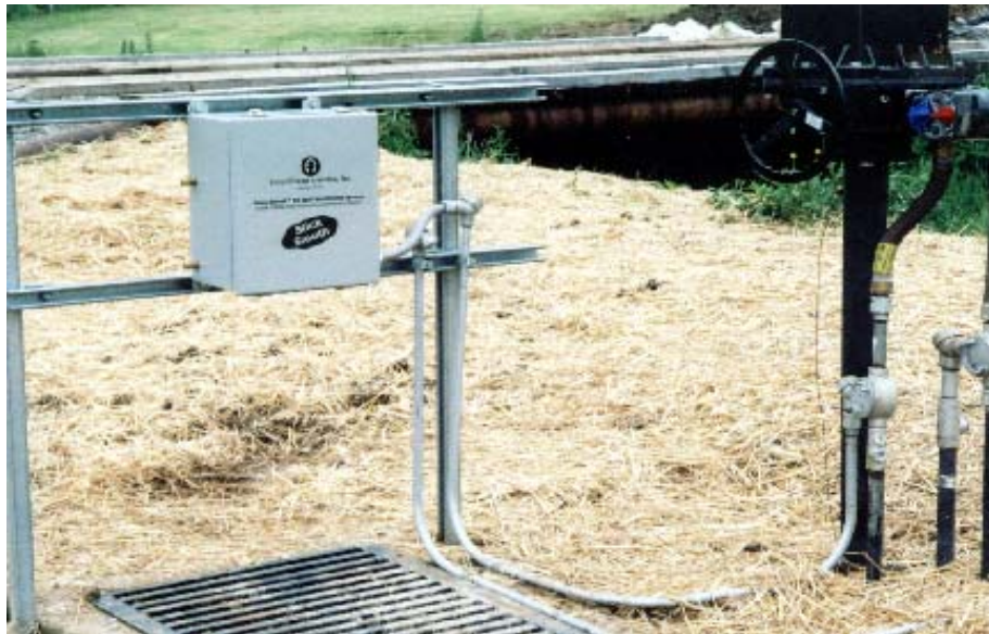
Figure 5. Oil detector operating over stormwater sump. Real time output to nearby control center, and automated shutoff of sump pump. Photo courtesy Dominion.
