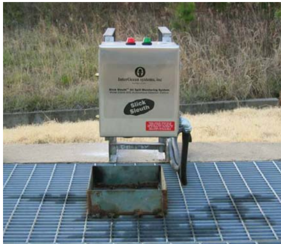
Figure 7. Unit deployed over deep sump at a GenCo in the USA. Automated control of sump pump discharge. Photo courtesy Entergy.
