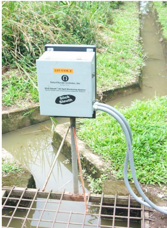
Figure 8. Discharge monitor installed at production facility in Ecuador. Photo courtesy Occidental.
