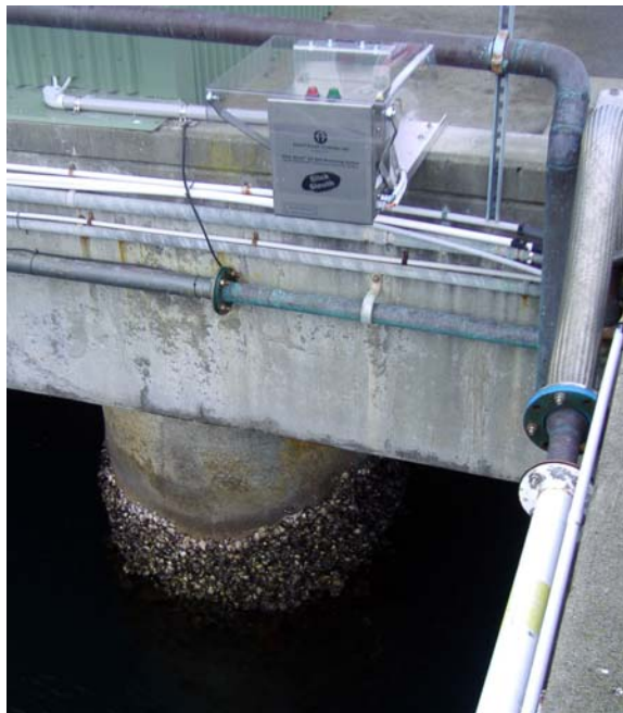
Figure 9. Slick Sleuth installed on fuel pier and marine terminal. Alarm output monitored using SMS messaging to key personnel. Photo courtesy RAN.
