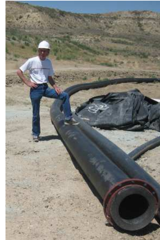
CBM Produced Water Gathering Pipes (WY)
